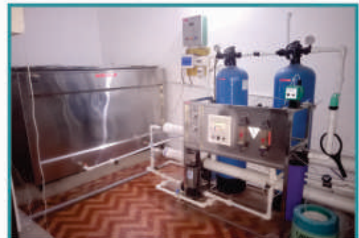
Water Treatment Plant With Chiller
